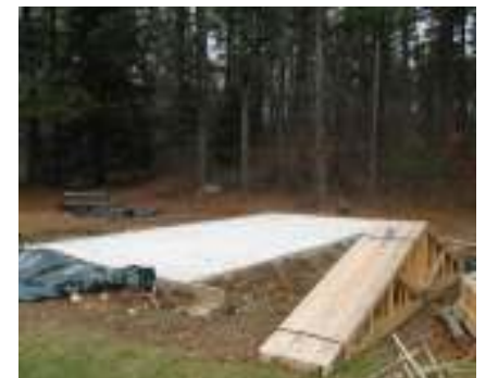
The concrete floor is poured; and lumber for the roof sits next to it, soon to be erected.
